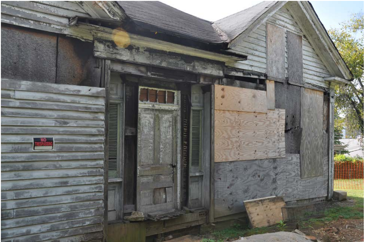
Picture #2 is a current view of the back side of the house. I have not done any work on it. There are two windows that were removed when the addition was put on back in the early 1920s that will have to be built and installed.
