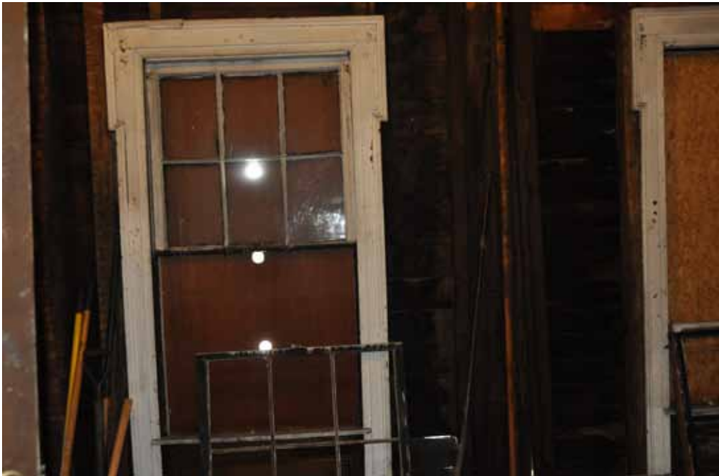
Picture #3 shows one of the 3 windows in the Dining Room. The window trim design is called "dog-eared" This picture also shows where I am removing the old sashes to be restored.
